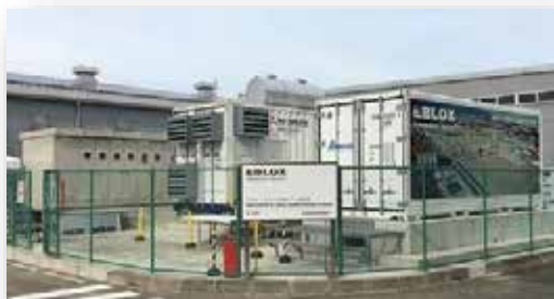
500kW/331kWh Sagamihara, Japan Micro-grid w/ PV, gas turbine
