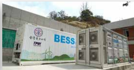
2MW/1MWh Kinmen, Taiwan Demand response, power backup, PV smoothing, frequency regulation
