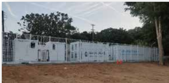
1MW/1MWh Changhua, Taiwan Peak shaving, power backup
