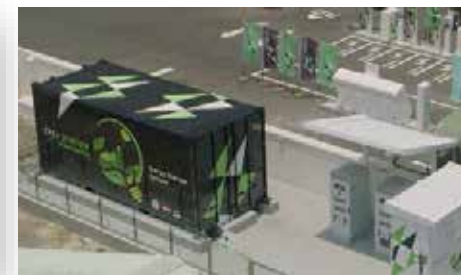
250kW/ 500kWh Chiayi, Taiwan Peak shaving, demand response w/ e-scooter charging station
